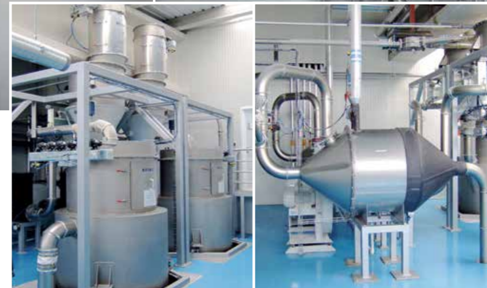
Flour cooling system
